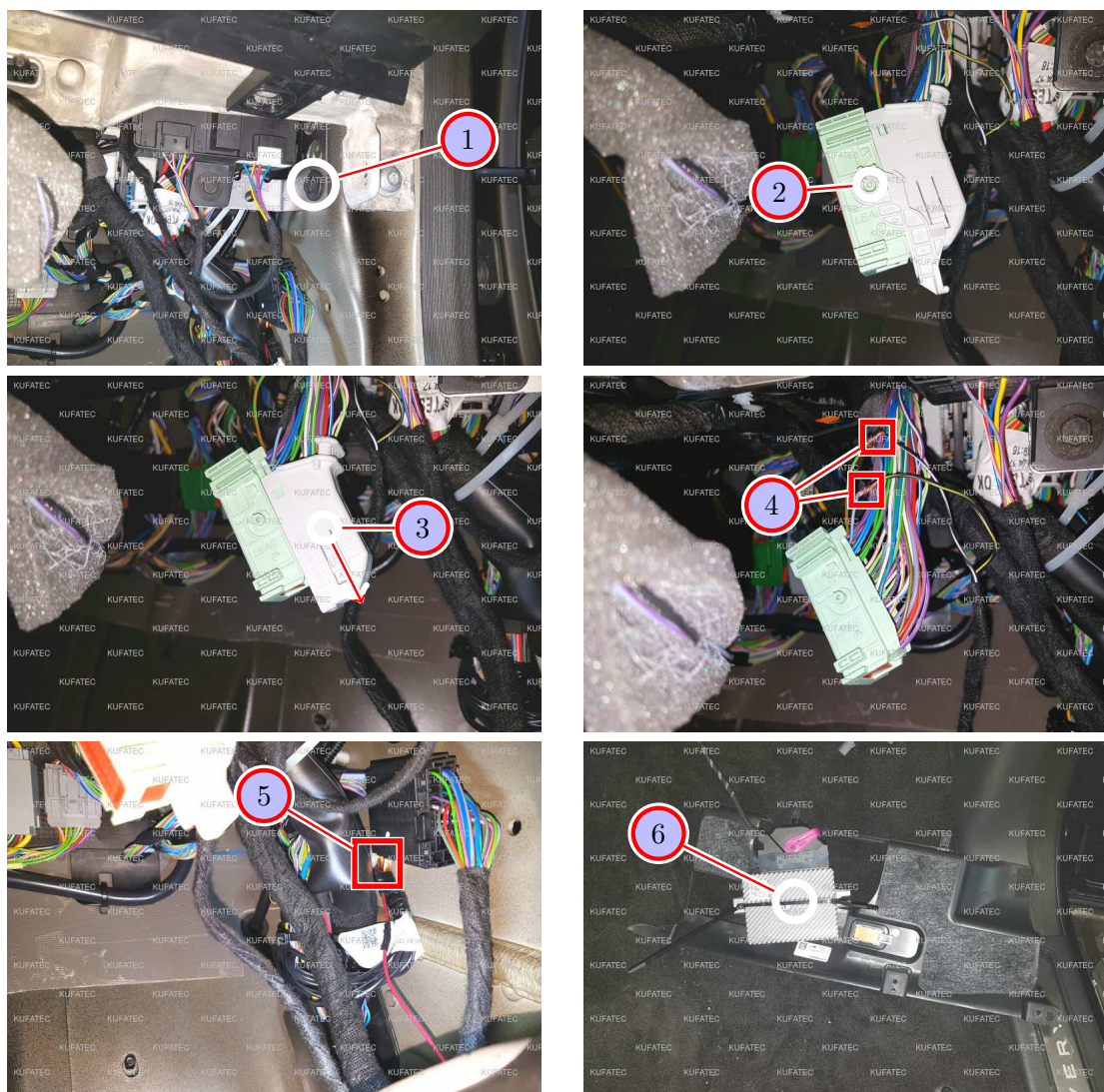
Figure 7: Connection cable set
